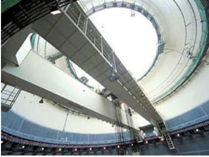
Polar Crane on the Rail
