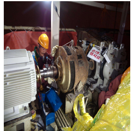
Align Main Hoist Motor
