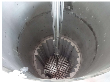
RM Mast Handling the Dummy Fuel in the Fuel Cell of RV Mock-up inside
