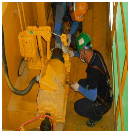
Replace Running Motor Brake
